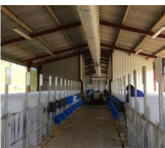
Positive pressure ventilation providing adequate air flow in the calf shed
