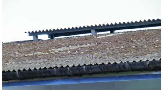
Raised ridge. Capping is fine as long as it does not restrict the ridge opening
