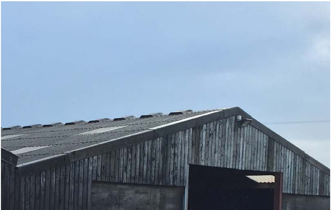
Ventilated ridge – inadequate. These ridges often supply less than 30% of the ventilation needs
