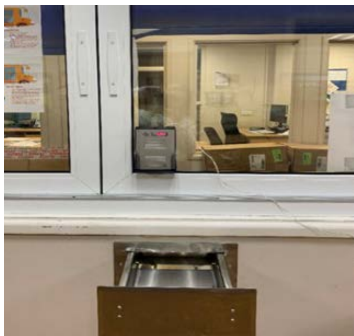
Figure 2. Example screened reception area and transfer drawer
