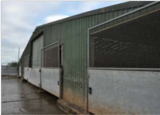
Plate 1. Ineffective mesh panels, gaps providing access in to building
