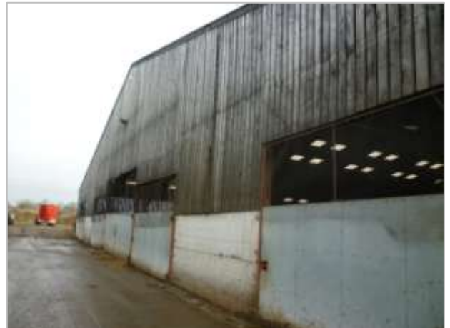
Plate 2. Effective netting applied to all openings including roof ridge
