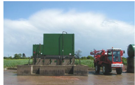
Compliant gravity fed system
