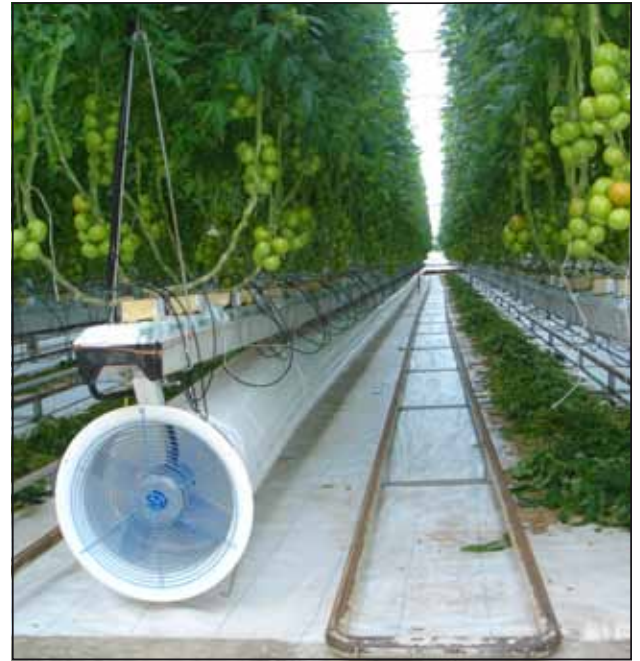
15 Use a fan and duct system or air circulation fans to minimise cold spots in a house
