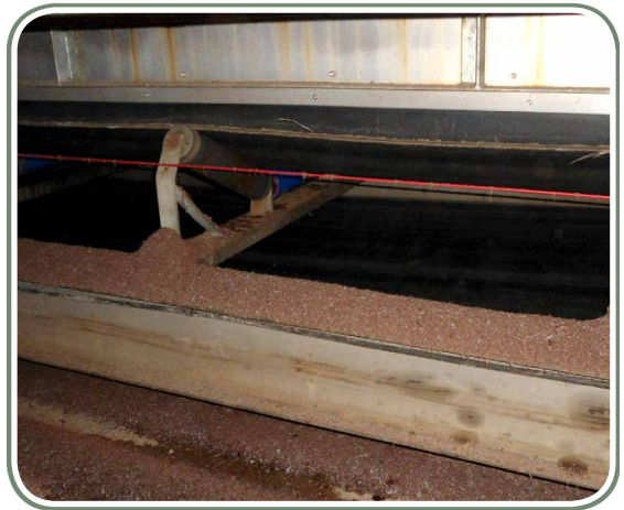
6. Debris build-up on conveyor during Phase 3 emptying
