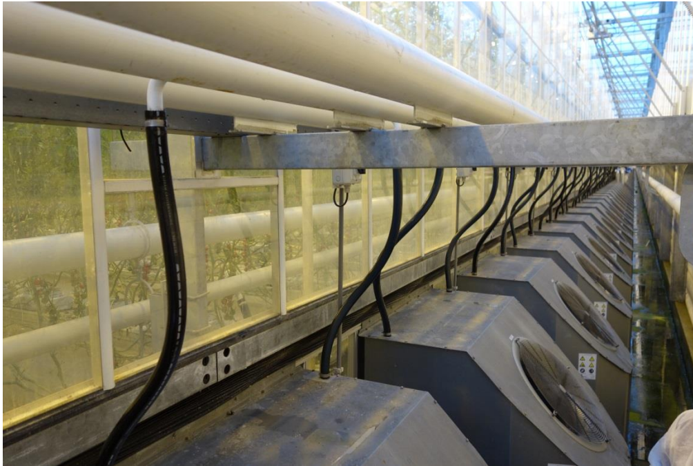
Figure 2: Forced air ventilation system in KUBO glasshouse
