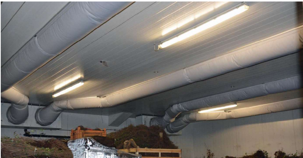
Figure 4: Air ventilation system
