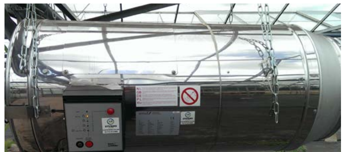
Figure 38. CO 2 burner (air heater)
