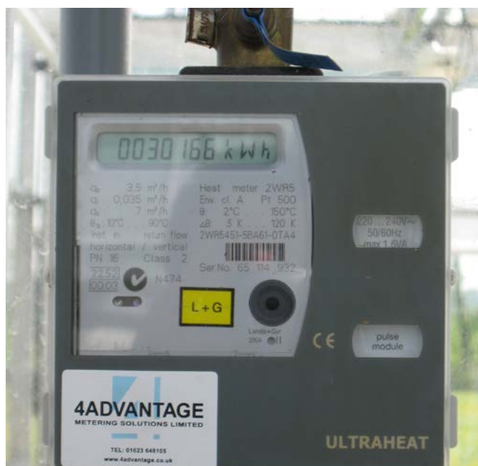
Figure 2. Meter used to monitor the heating energy used in a specific greenhouse area
