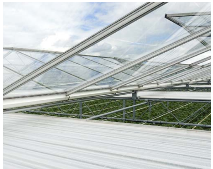
Figure 31. Screen gapping and venting in operation
