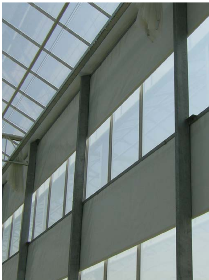
Figure 60. Side screens can reduce horizontal temperature stratification and save energy
