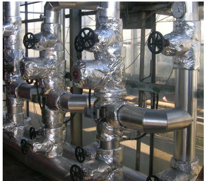
Figure 10. A good example of how flexible jackets can be used to insulate pumps and valves
