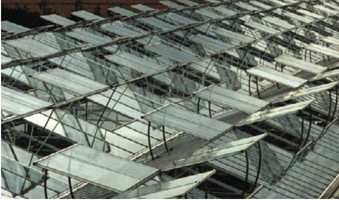
Figure 23. Venting results in energy loss but is an essential element in humidity control
