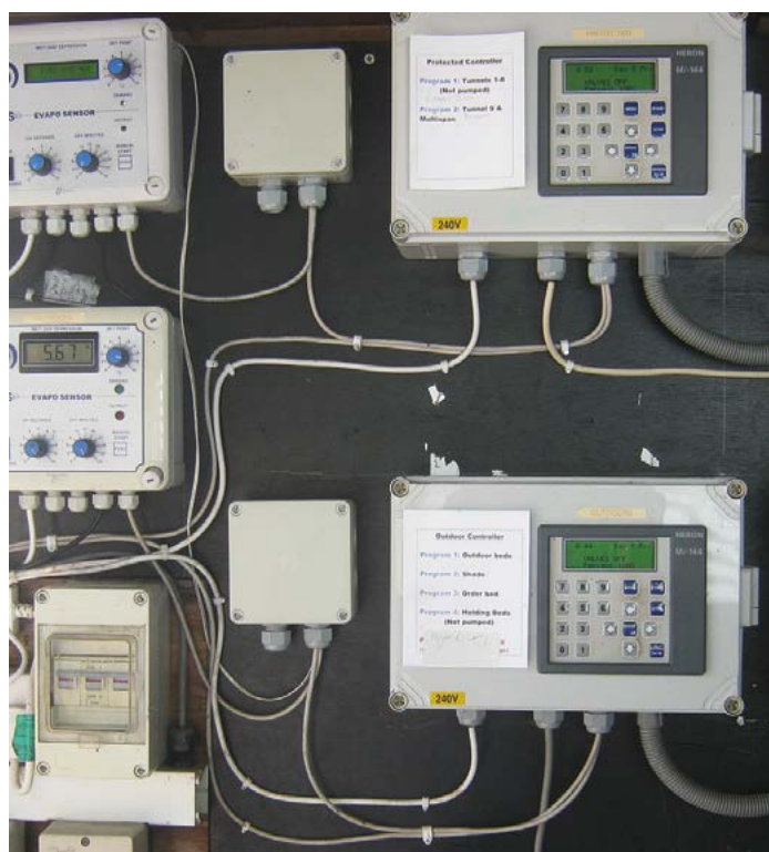
Figure 8. Evapotranspiration monitoring equipment linked to irrigation control panels
