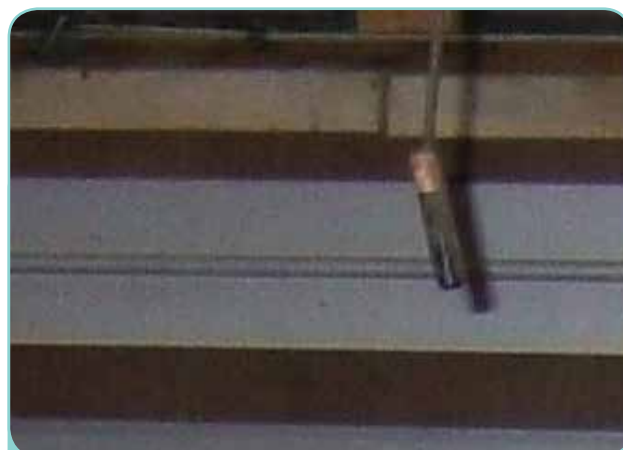
Temperature sensor incorrectly located by a vent
