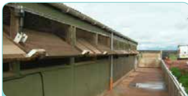
View of the main vents from the outside
