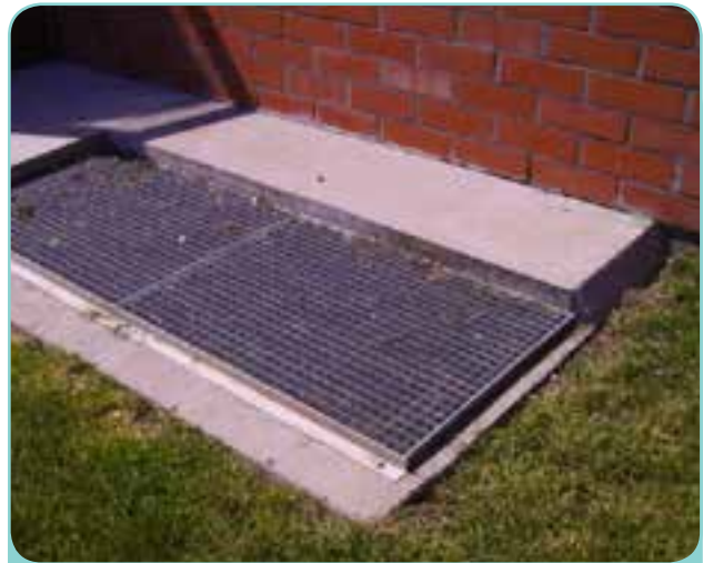
Under passage ventilation inlet
