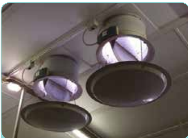
Roof mounted exhaust ventilation fans showing control flap within the chimney. Also shown is the rain trap dish below the fan chimney.
