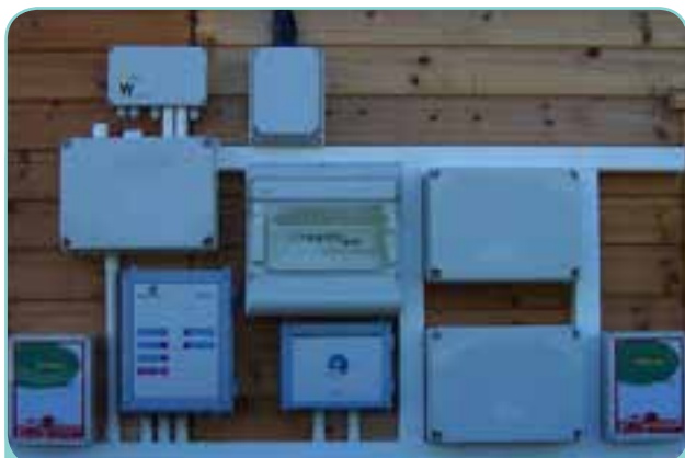
Ventilation control computer and other electrical panels
