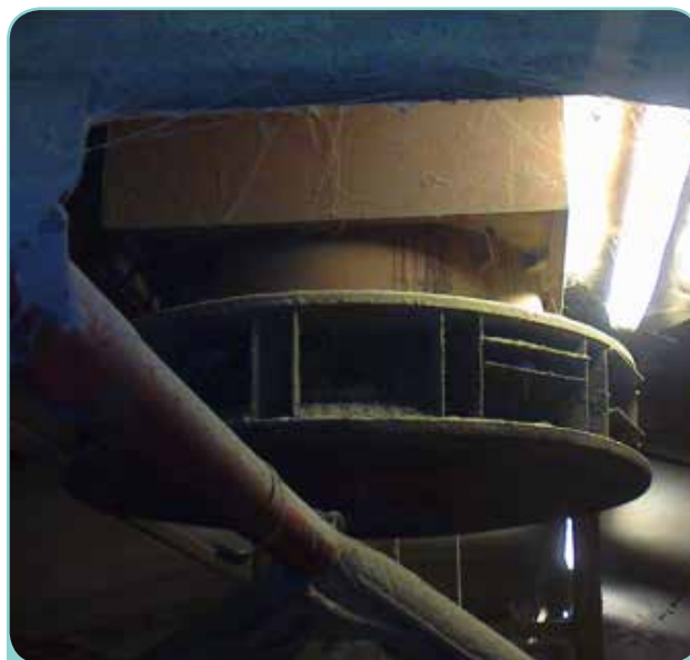
Pressurised recirculation unit
