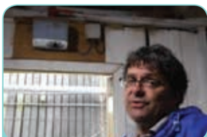
Motor and winch limit switches
