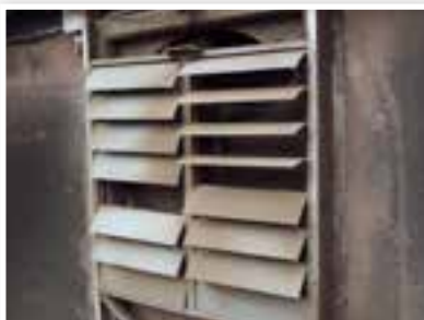
Broken flaps are a common maintenance fault
