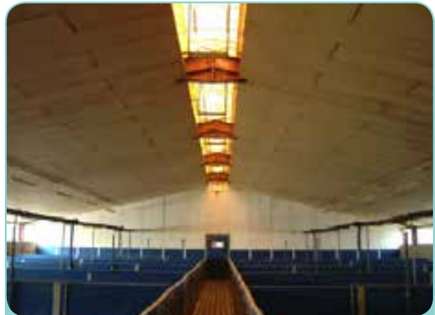
Controlled ridge ventilation in a fully slatted building
