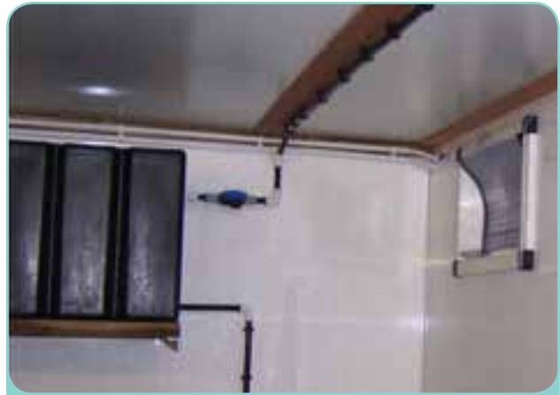
A water tank and supply pipe which could affect the airflow from the adjacent inlets
