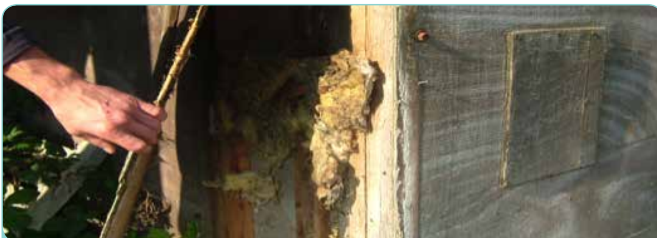
Insulation damaged by rodents
