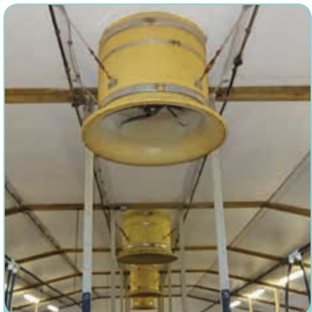
Ridge extraction fans in the roof
