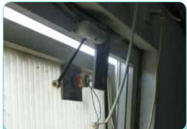
An emergency ventilation drop-out panel controlled by an electromagnet
