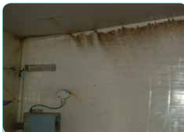
Draughts are entering the building along the junction of the roof and the side wall
