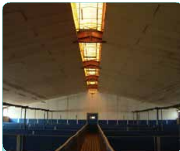
The inside of a building with both automatic ridge and side-to-side ventilation
