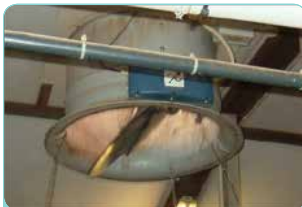
Exhaust fan chimney fitted with a control flap. Both fan speed and degree of flap opening are controlled by a computer to ensure the room is maintained at the optimum temperature for the age and category of pig housed
