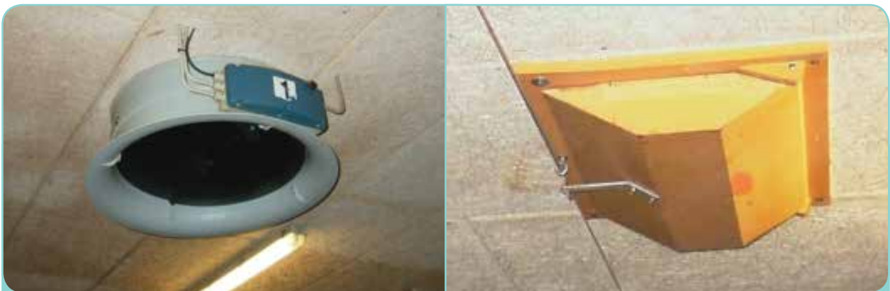
Danish permeable ceiling showing a fan (left) and air inlets (right)
