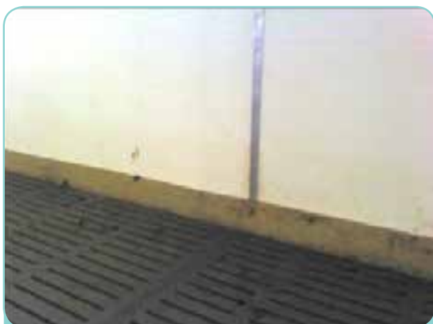
Photograph of a concrete fillet which is acting as a thermal bridge
