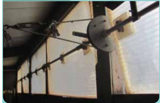
View of the inside of a modern monopitch building showing the front and rear vents and the rope and pulley system linking them
