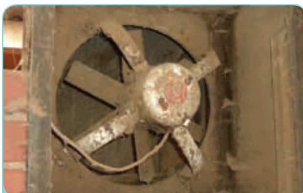
Very poorly maintained fan
