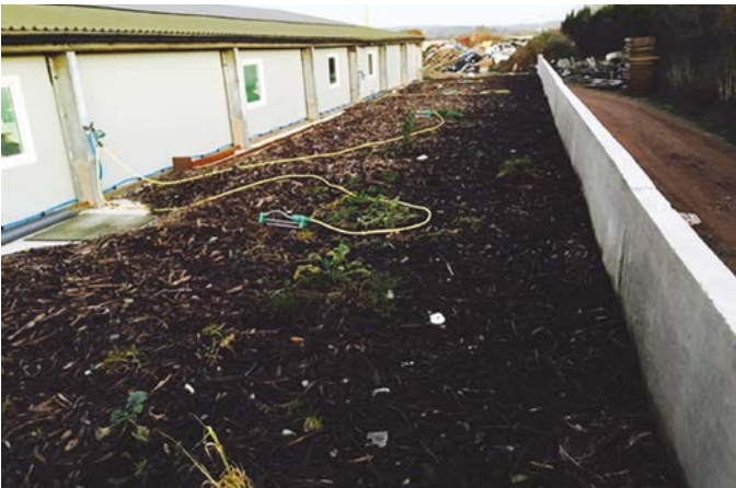
Figure 37. Biofilter with wood chippings/bark as a base
