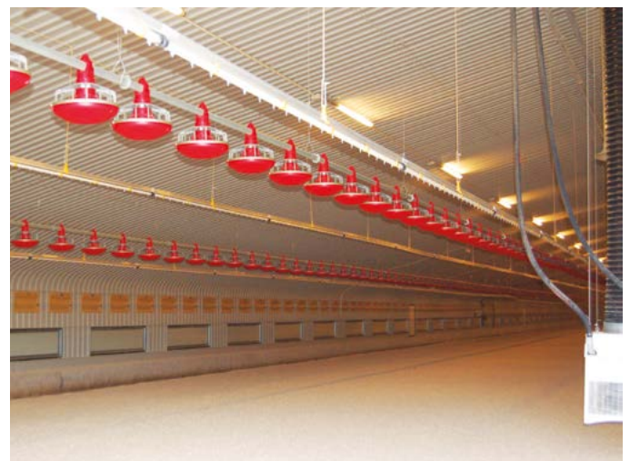
Figure 88. Lighting in a broiler building
