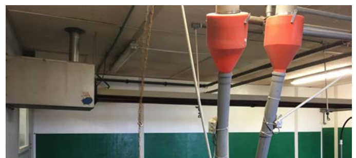
Figure 74. Radiant gas heater pipes
