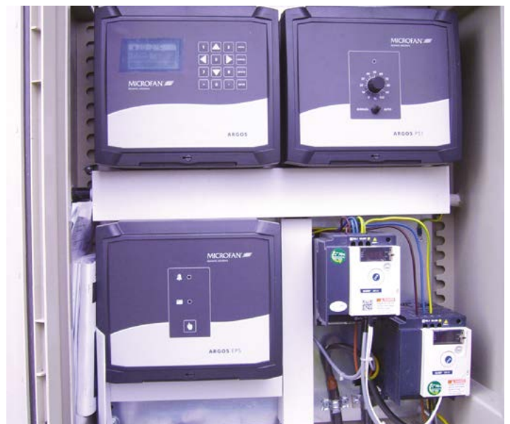
Figure 83. Modern controller interface
