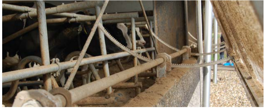
Controlled window air inlets – cattle housing
