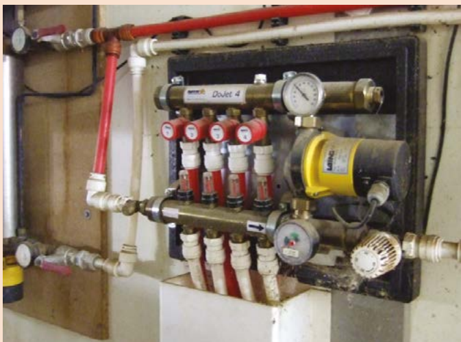
Figure A1.1 Control valve manifold for wet heating system
