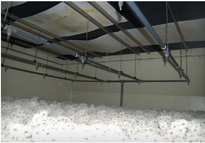
Figure 36. Chemical spray bars and media – acid wash air scrubber
