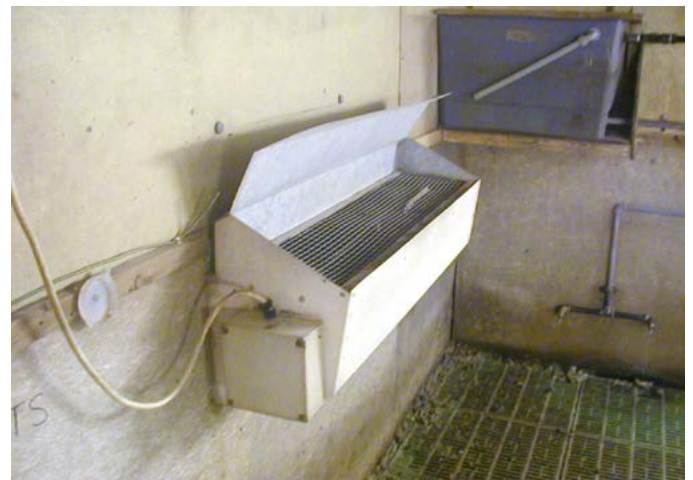
Figure 64. Heated inlet duct
