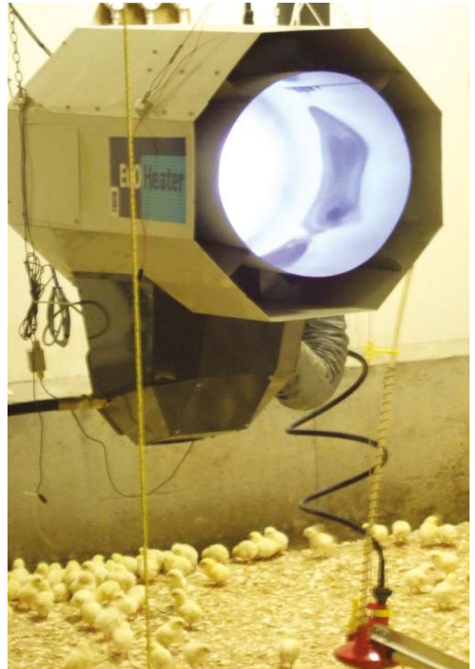
Figure 16. Badly maintained gas heaters can produce carbon monoxide
