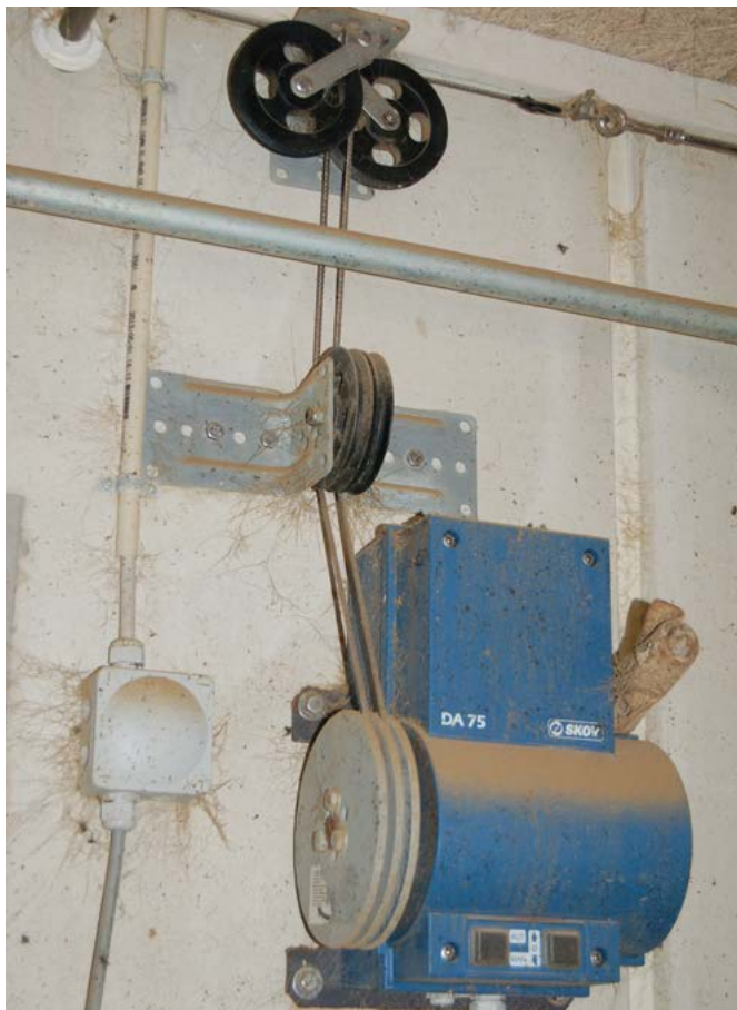
Figure 98. Winch and pulleys controlling ventilation inlet opening in proportion to fan speed
