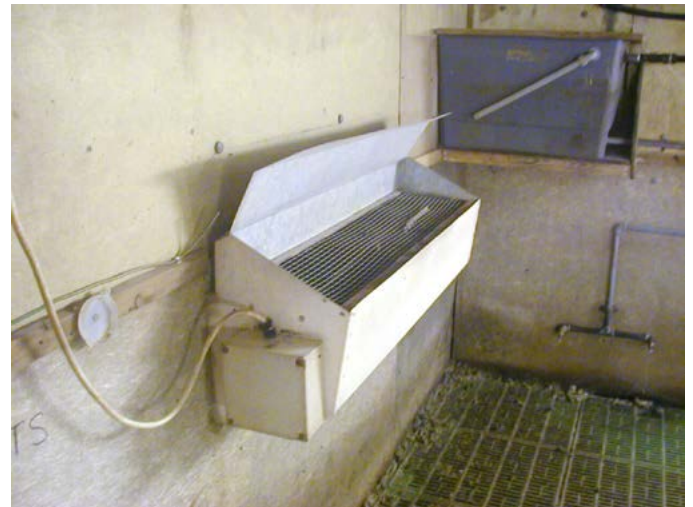
Figure 73. Duct heater in weaner room
