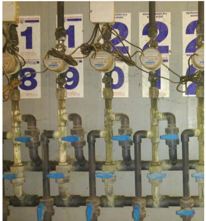
Figure 4. Water distribution manifold for fresh drinking water, medicated water and line cleansing
