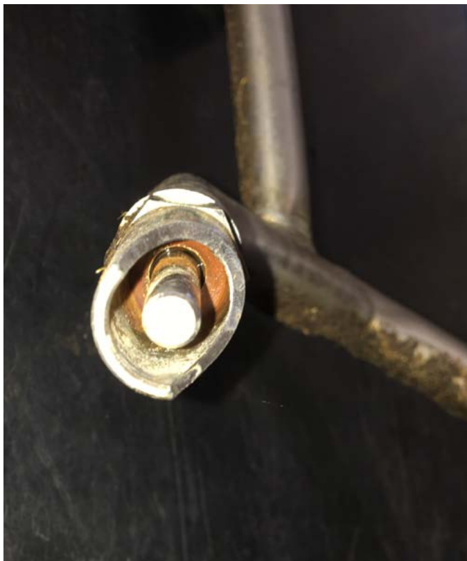
Figure 2. Biofilm build-up inside a water pipe after one batch of pigs
