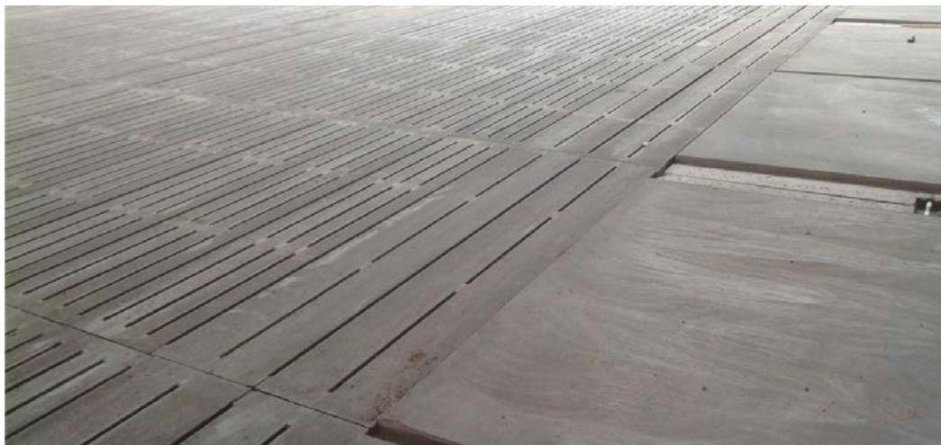
Figure 6. Finished room with under-slat cooling and heated lying areas
