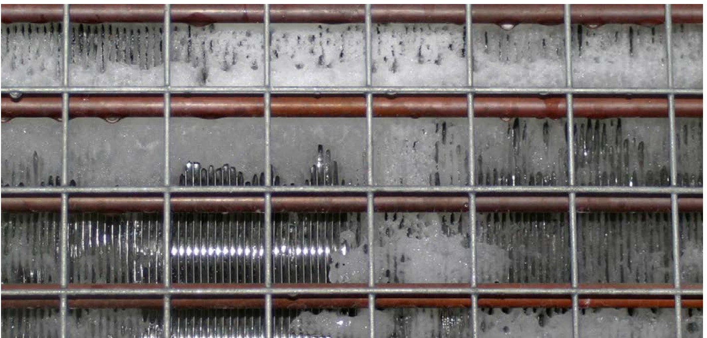
Figure 21. Ice must be regularly cleared from cooling coils
