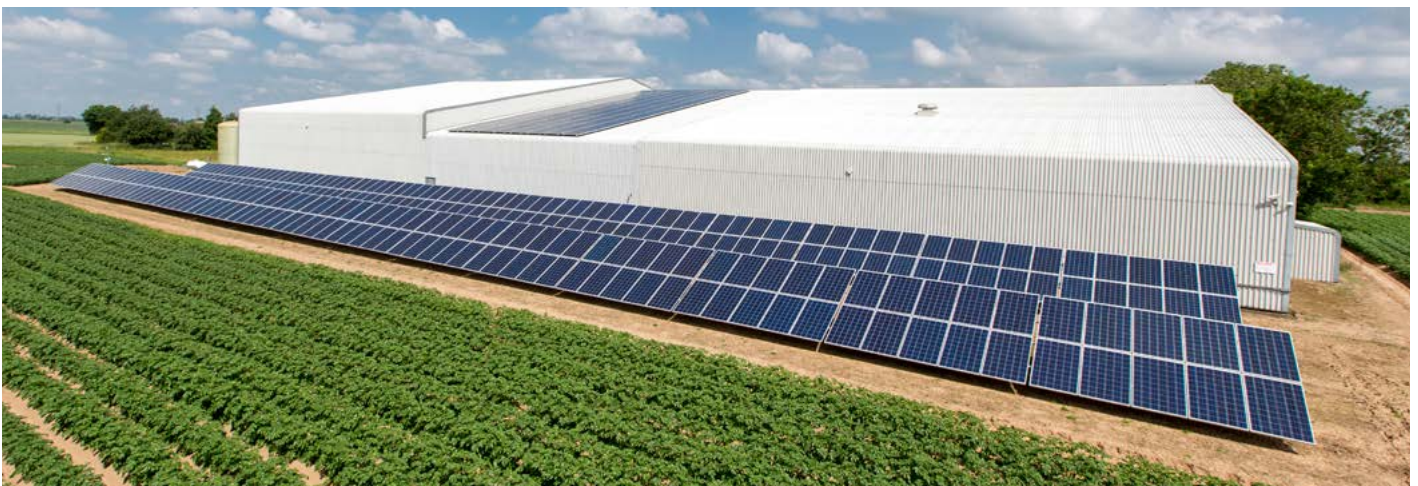
Figure 26. Refrigerated potato stores can make good use of solar energy in summer months
