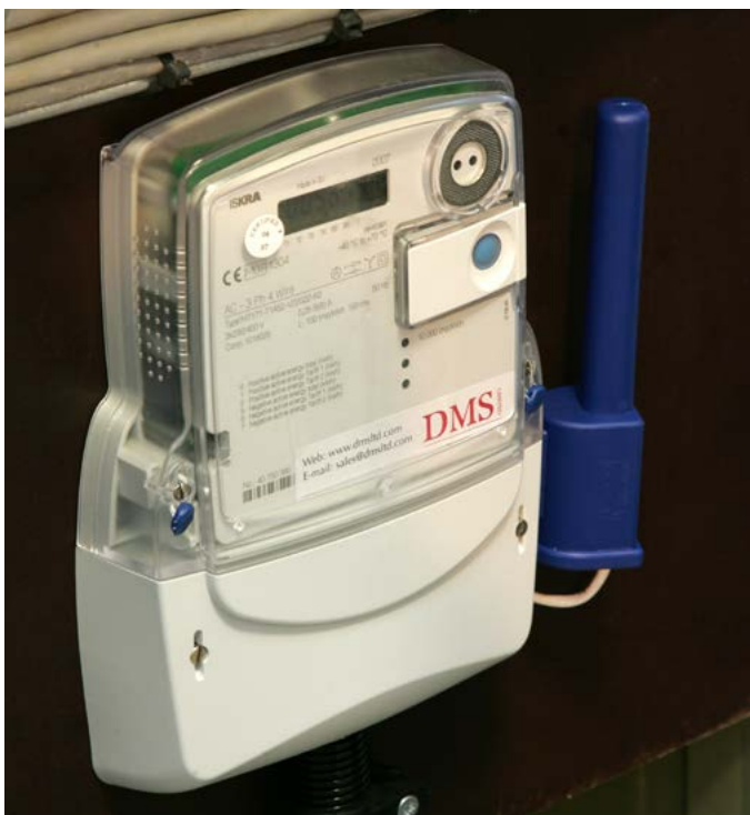
Figure 23. Store-specific smart meter
