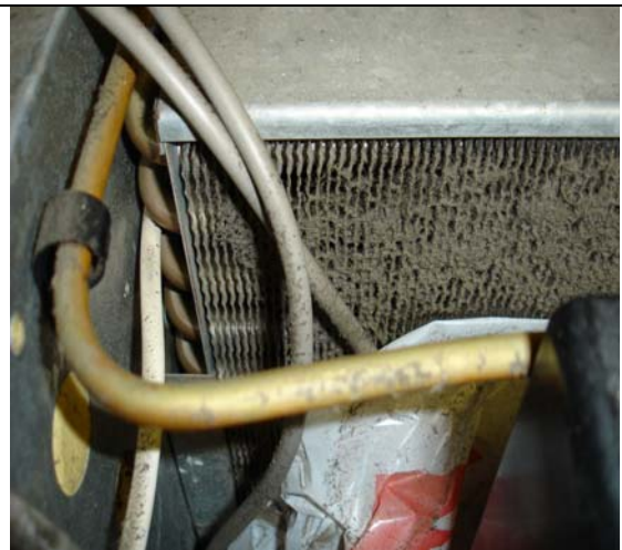
Figure 10 A dirty Condenser with plastic bag blocking free flowing air
