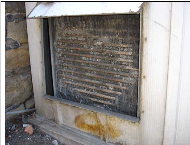
Figure 9 Condenser on the verge of failing
