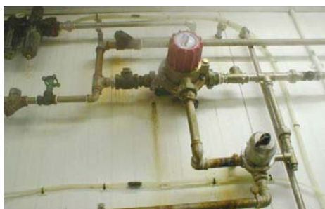
Pipework with no labelling or arrows denoting direction of flow
