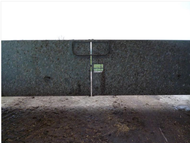
Heavy fouling on gates
