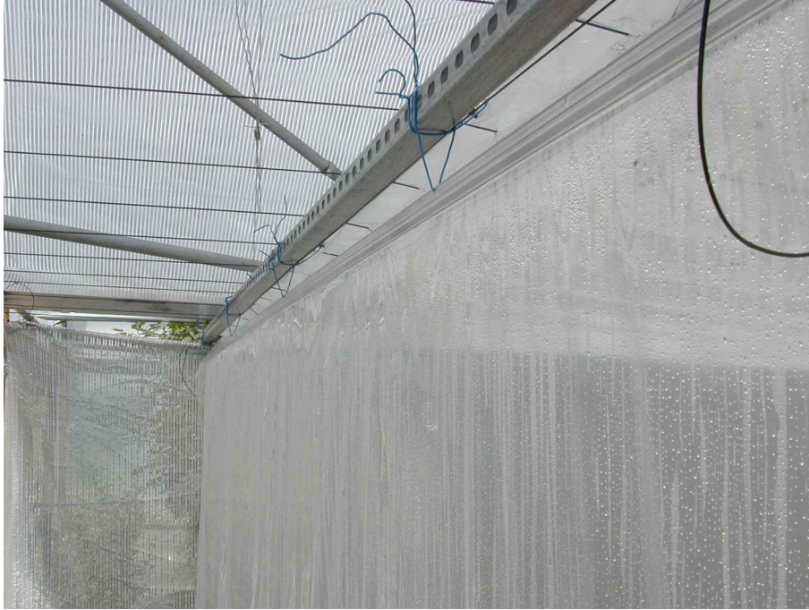
Plate 3. One wall of the large enclosure, showing the use of V-Grip to suspend the polythene from the supporting framework and to apply tension.
