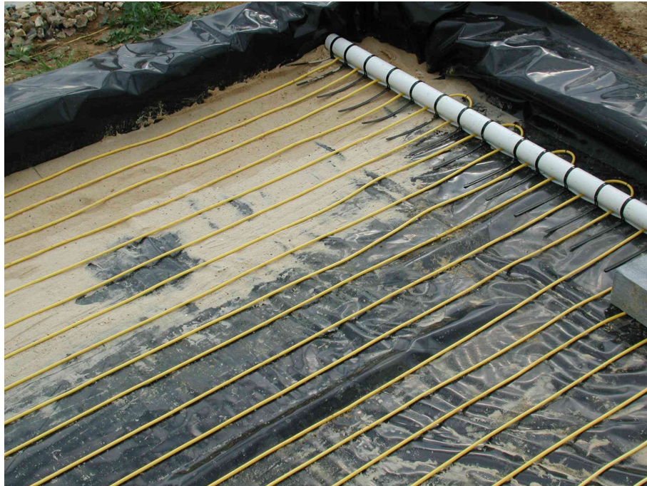
Plate 17. Construction of the propagation bed for the large-scale enclosed mist. The photograph shows the polythene liner, which covers a layer of expanded polystyrene sheets, and, on top of the polythene, the heating wires, which are held at the correct spacing by a former made from PVC pipe. Annual report Feb, 2002
